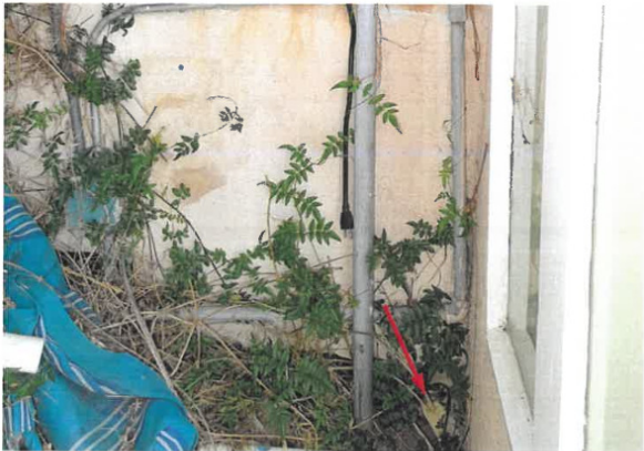
Debris filled drain exit at base of west side drainage channel behind retaining wall adjacent to first floor office/bedroom.
