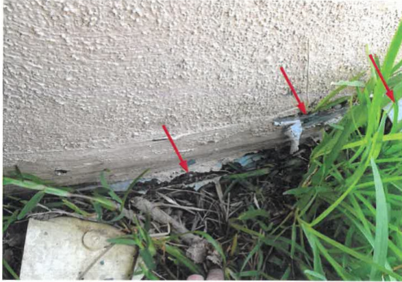
Exposed foundation waterproofing membrane at first floor south of retaining wall, note separations and exposed pipe.
