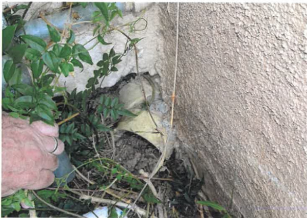
Close-up of debris filled drain exit at first floor west side exterior wall.
