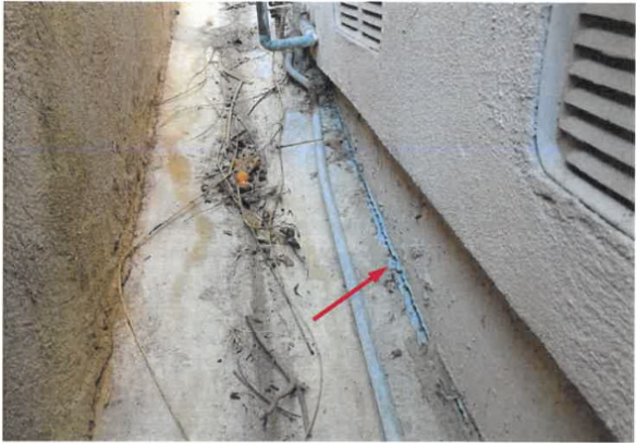
Close-up of drainage channel, note separation and sealant/patching materials.
