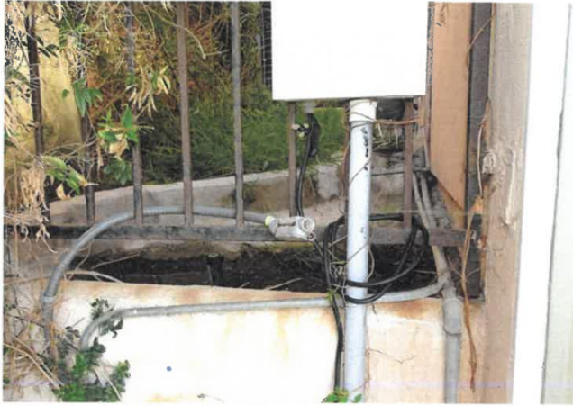
Debris filled drain at base of west side drainage channel at first floor office/bedroom exterior wall.
