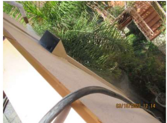
21 IMG_4754 – Wand test – leak in less than 5 minutes.
