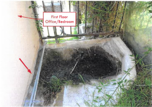
West side exterior wall at base of drainage channel, note debris filled drain, standing water and separation between retaining wall and drainage channel.
